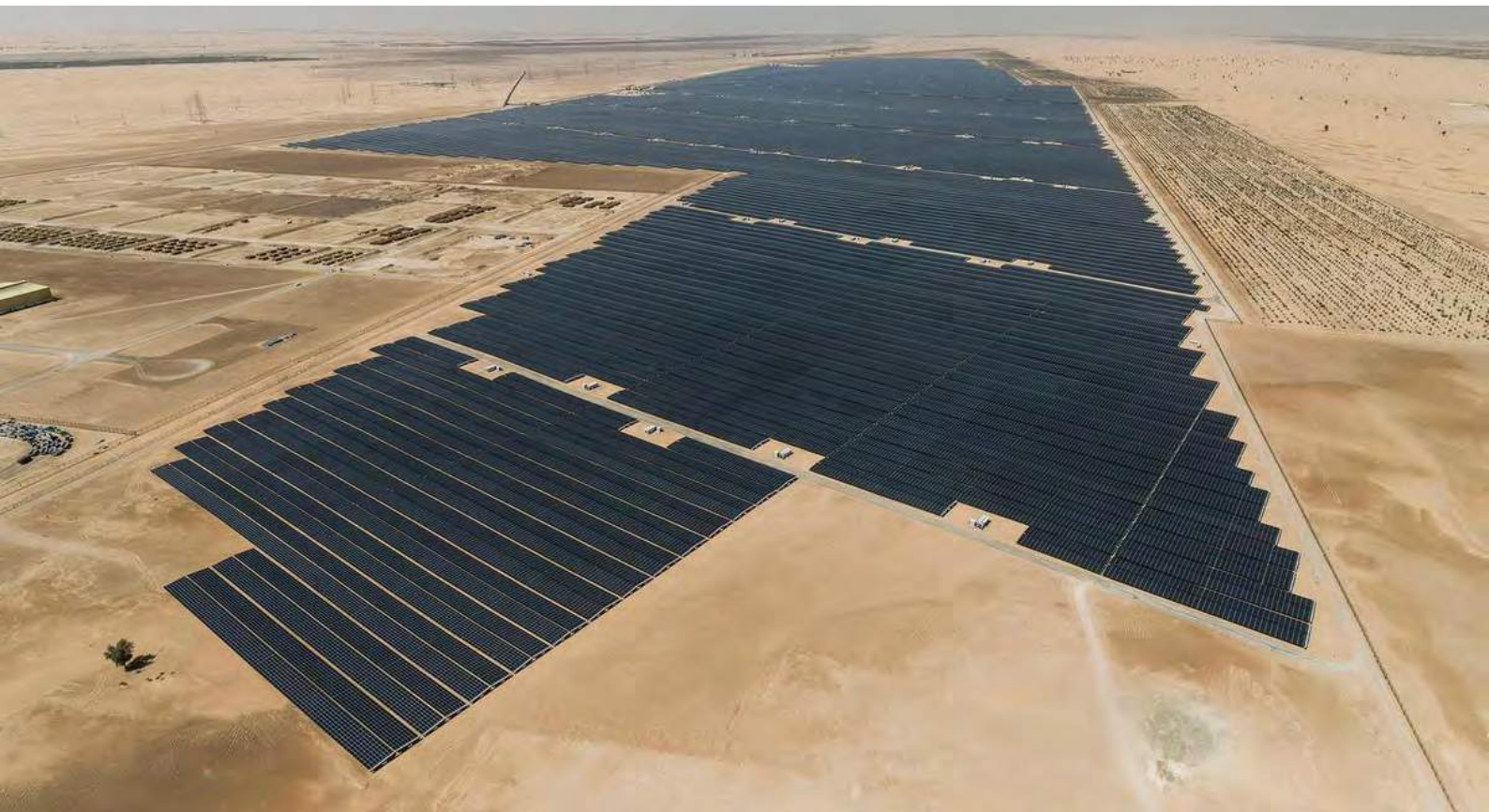
Noor Abu Dhabi solar plant, UAE
